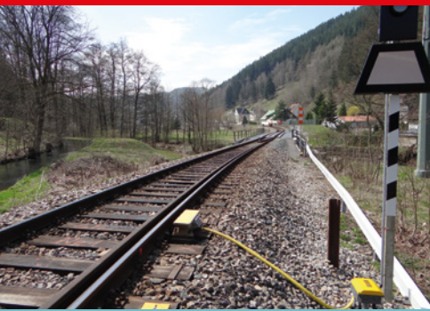
Wayside control track magnet
